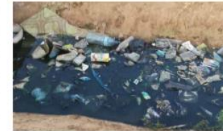
Waste clogging drainage channels
