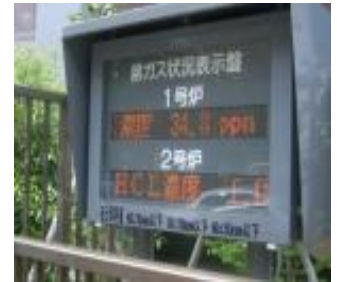
Incineration plants display gas status on a display in real time (Setagaya Incineration Plant)
